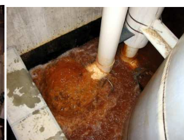
Backwash – Iron Removal
